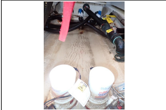
Aft Bilge Pumps
