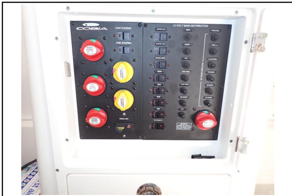
Main Battery switches
